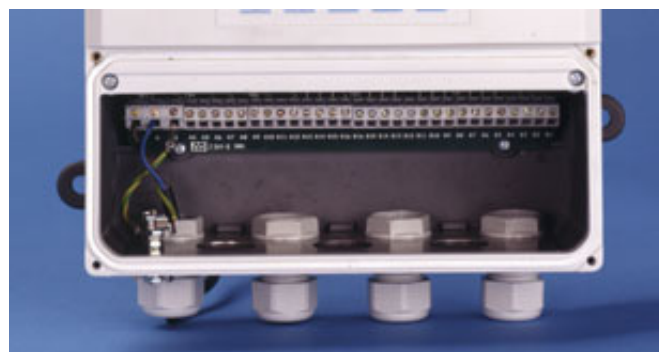
AV400 Termination Chamber Makes Access Easy
